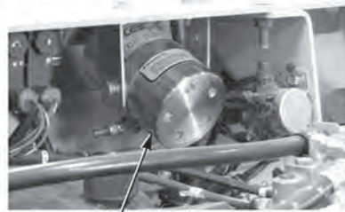
DRIVER SIDE FIREWALL AEROSOL GENERATOR
