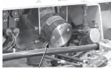
DRIVER SIDE FIREWALL AEROSOL GENERATOR
