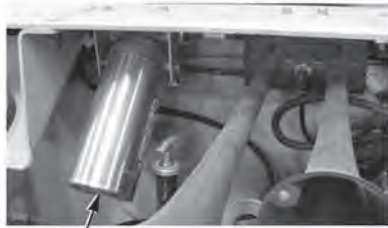
PASSENGER SIDE FIREWALL AEROSOL GENERATOR
