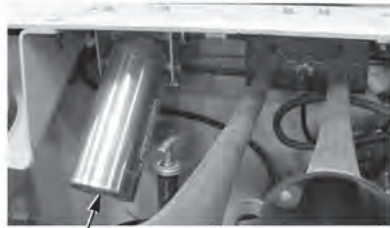
PASSENGER SIDE FIREWALL AEROSOL GENERATOR
